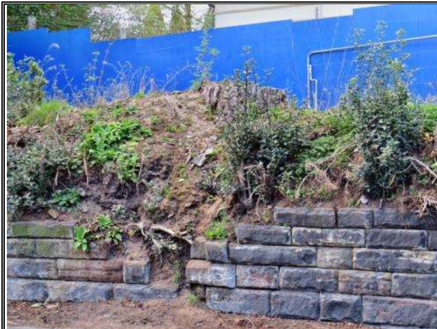
Photograph 163: Damage to Boundary Wall from Tree Growth
