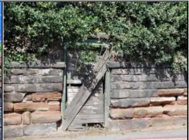
Photograph 164: Boundary Wall and Door in Poor Repair
