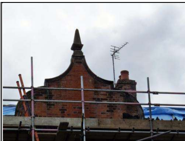
Photograph 135: Restoration of Bank Hall, Stamford Road, for Continued Usage as a School
